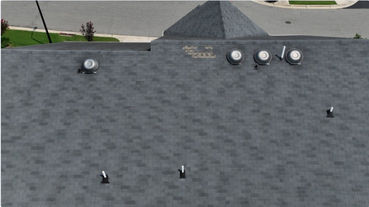
Fig. 2 — Missing shingles along the upper ridge, underlayment exposed across the affected courses.
