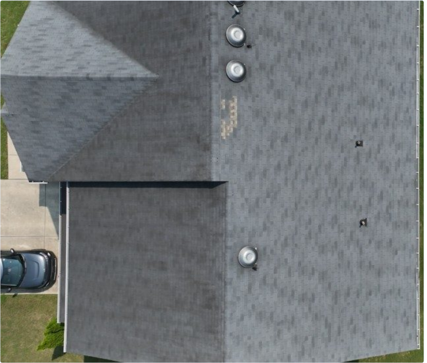
Fig. 3 — Closer pass on the same area; extent of exposure and boundary of the affected courses.
