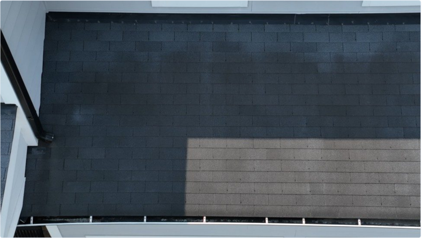
Fig. 6 — Valley transition and gutter line. Localized surface discoloration noted as a LOW observation.
