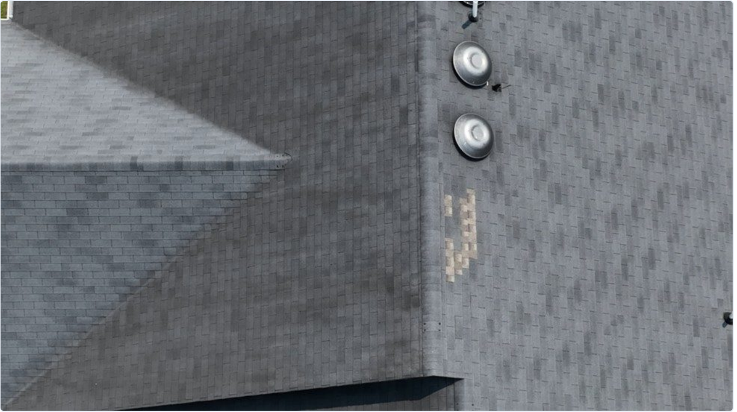
Fig. 4 — Same finding from the opposing approach. Two angles on one defect.
