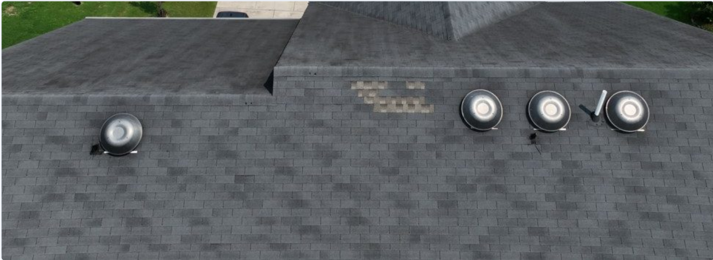
Fig. 1 — Upper south-facing plane. Affected area sits immediately below the ridge; surrounding field, vents and ridge line intact.
